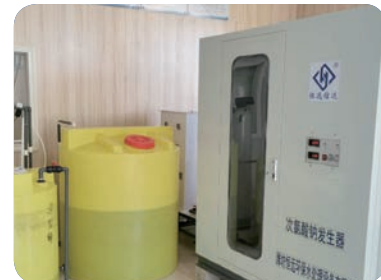
Xingyi Water Treatment Plant Project, Guizhou
