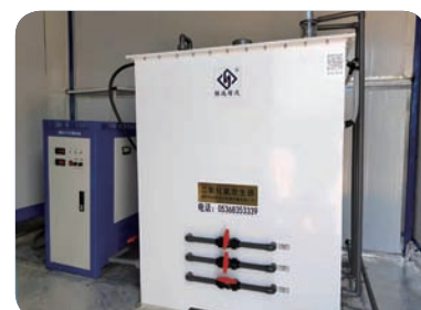
Jilin Songyuan Water Treatment Plant Project
