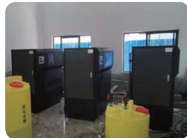
Hebei Gu'an Water Treatment Plant Project
